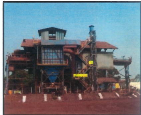
Dust Extraction System at
