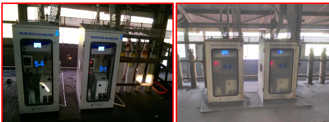
Continuous Emission Monitoring System
