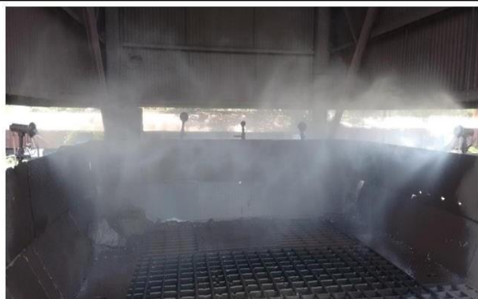
Dry Fogging System for Fugitive dust suppression
