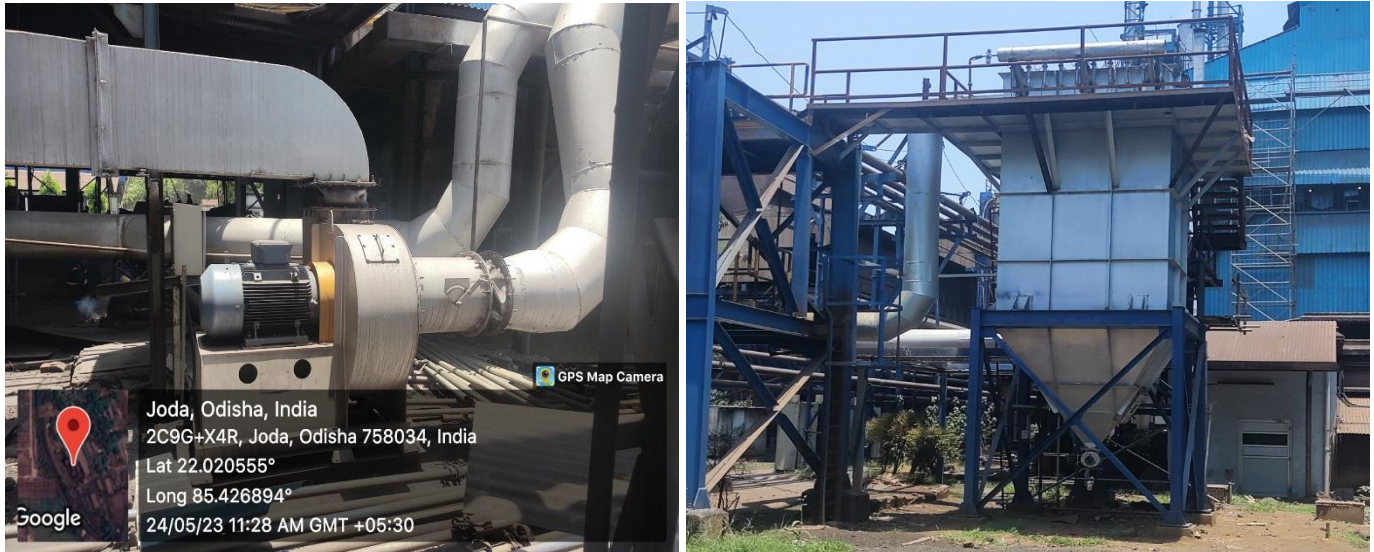
New Fume extraction system with bag filter
