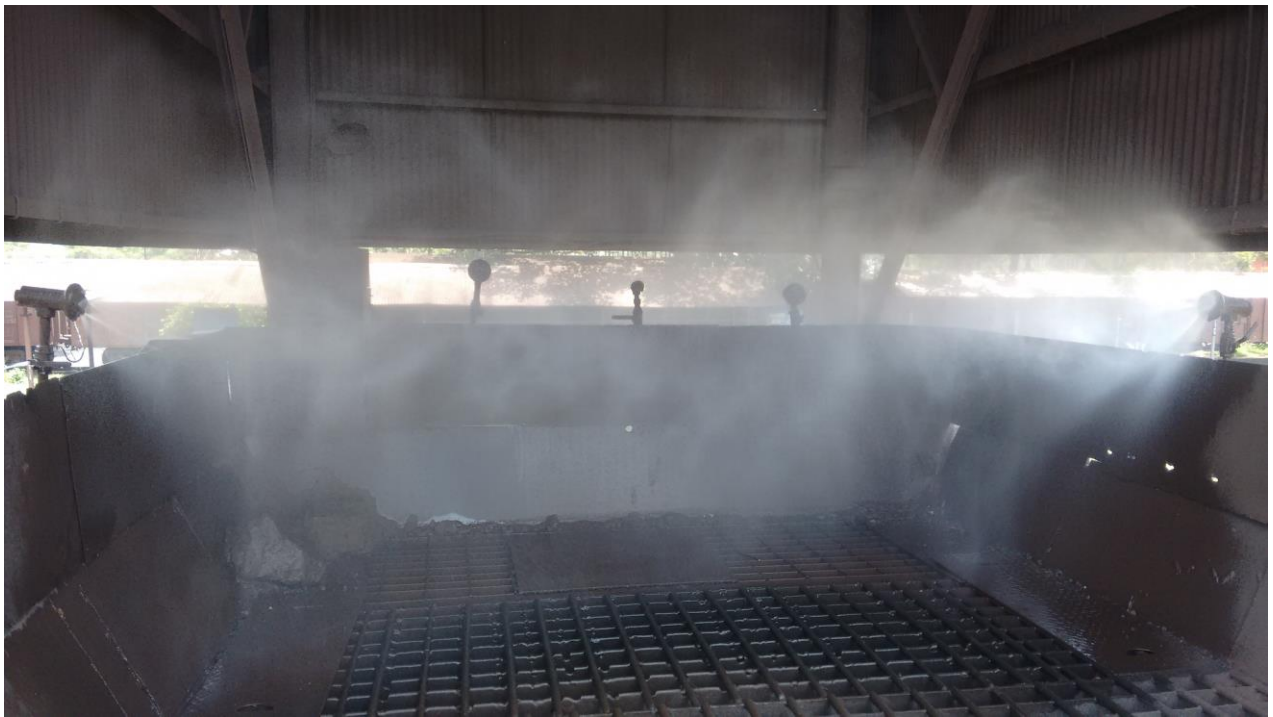
Dry Fogging System for Fugitive dust suppression
