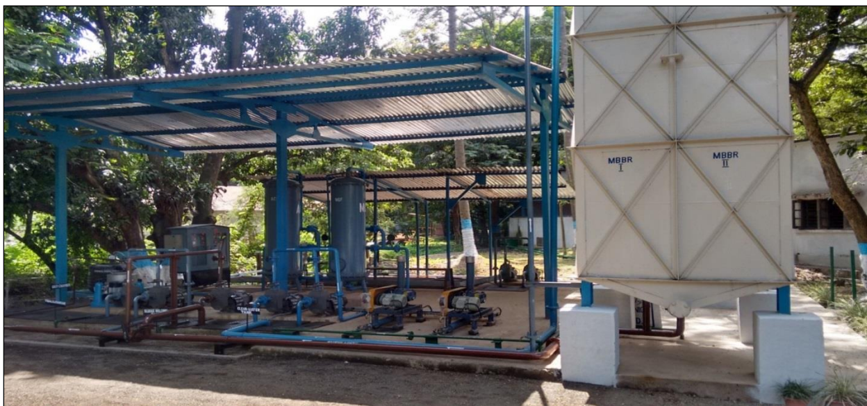
Sewage Treatment Plant Installed at FAP, Joda
