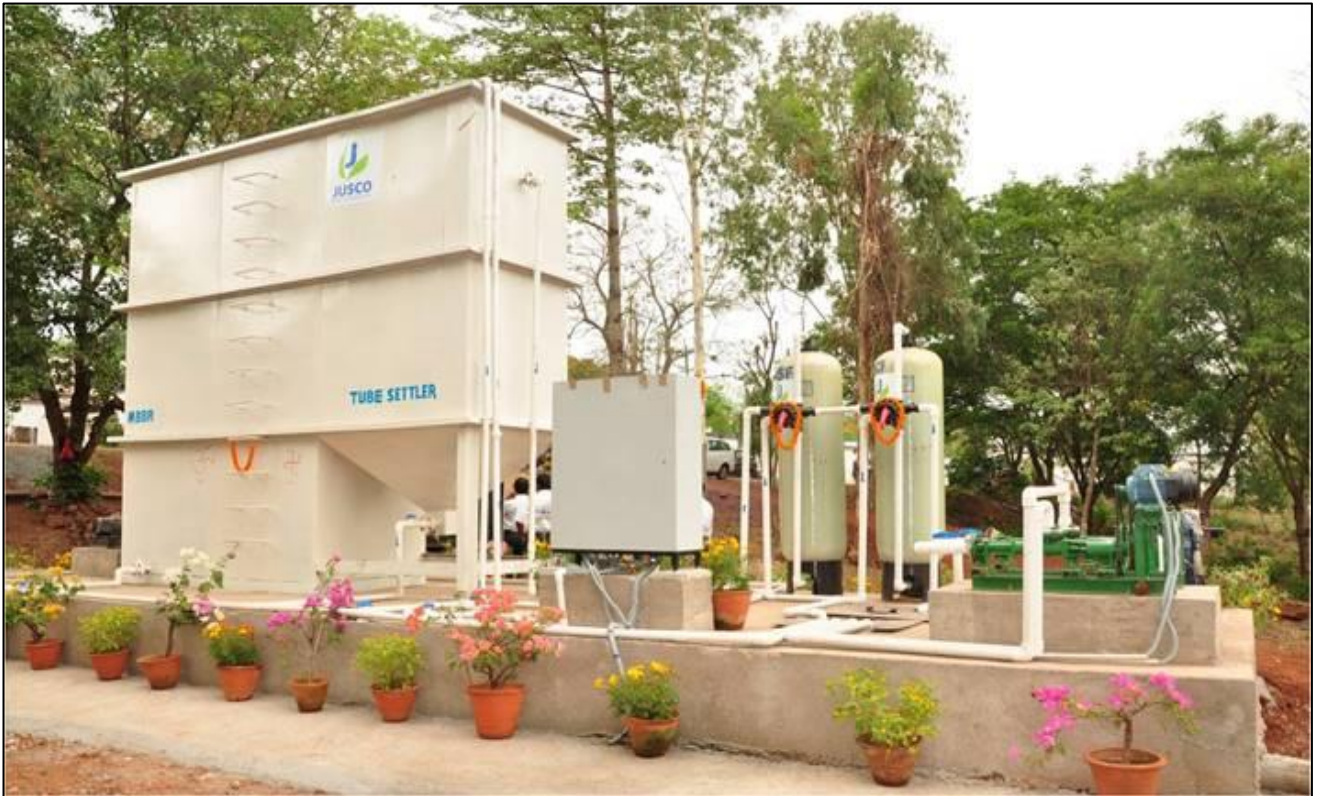
Sewage Treatment Plant
