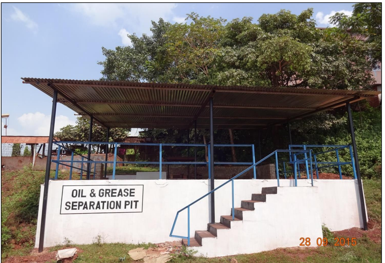
Oil & Grease Separation Pit
