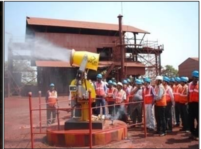
Water Mist System in Plant
