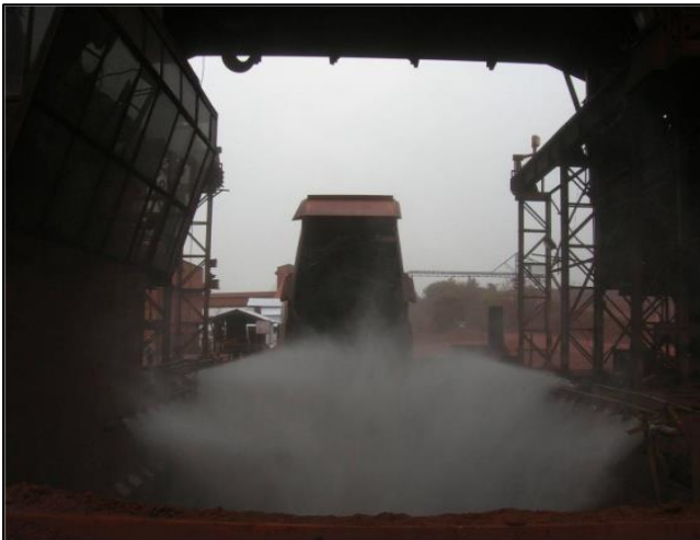
Water Jet System at Unloading Point
