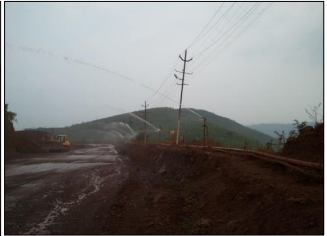
Fixed Water Sprinkler
