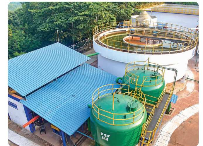
Water treatment plant at Noamundi, Jharkhand
