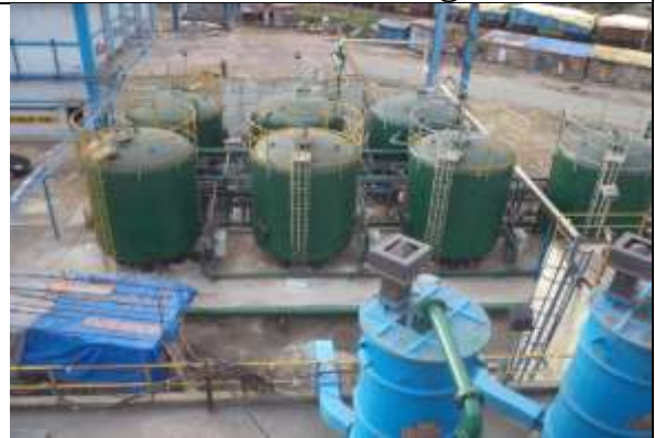
Side stream filter of CETP
