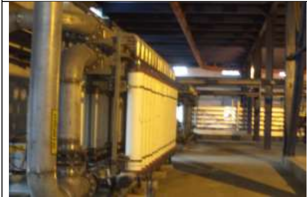
Reverse Osmosis Plant
