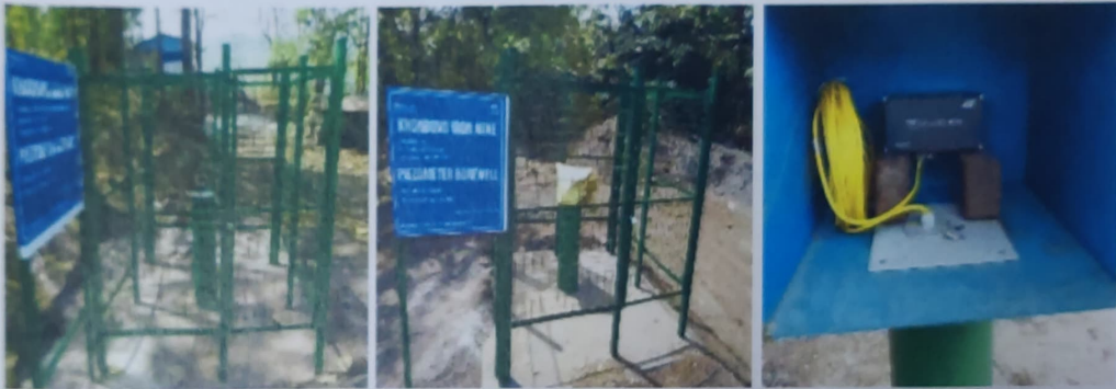
Piezometer (STP and Manganese) with digital recorder
