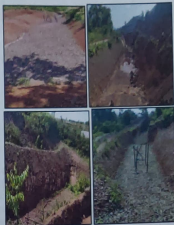
Four number of recharge pit with bore hole
